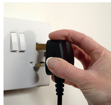
FIGURE 2.6.17d: Each socket has 230V applied to it.
